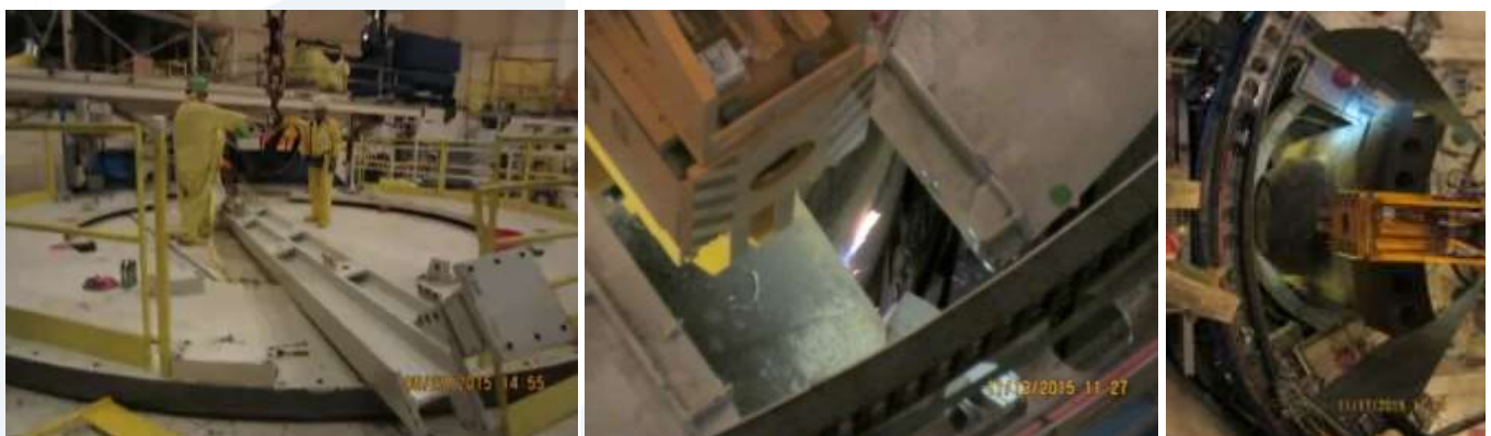
Figure A6.1. Contamination Control for Zion NPP RPV segmentation. Top part of confinement (left), ventilation of opening while cutting (center), and cut piece removal through opening (right) [Ref. 11]
