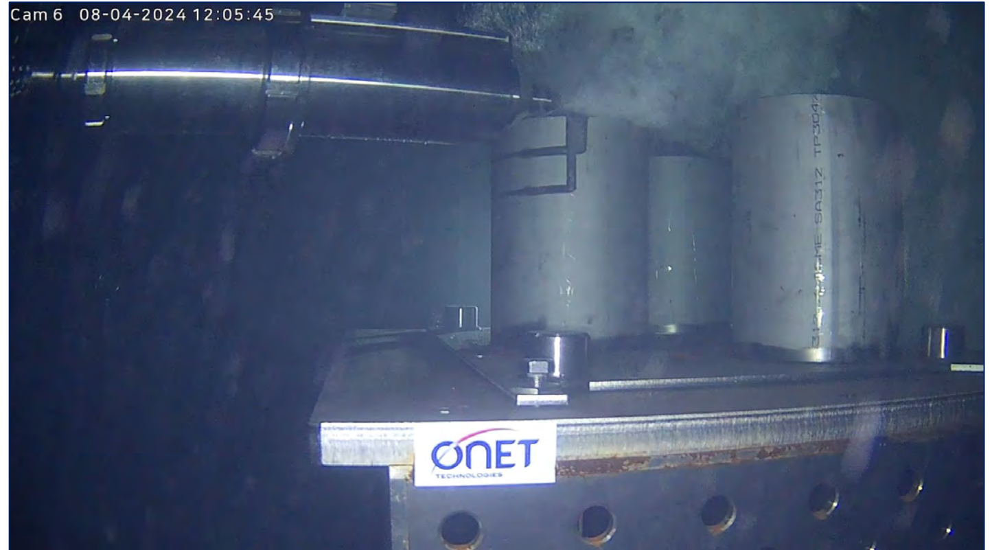
Underwater cutting of mock-up (BWR Poisoning plate) at Onet Technocenter. Source: Onet.
